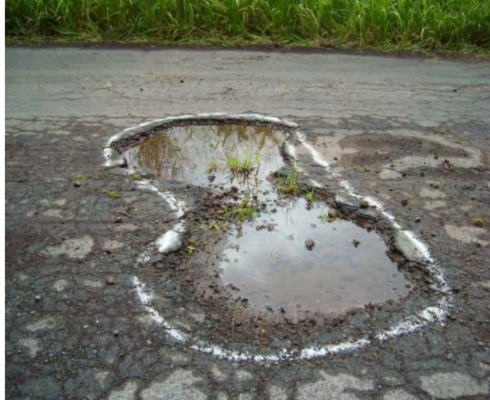
5 Figure 9: Potholes forming due to lack of maintenance on Ka'alāiki Road
